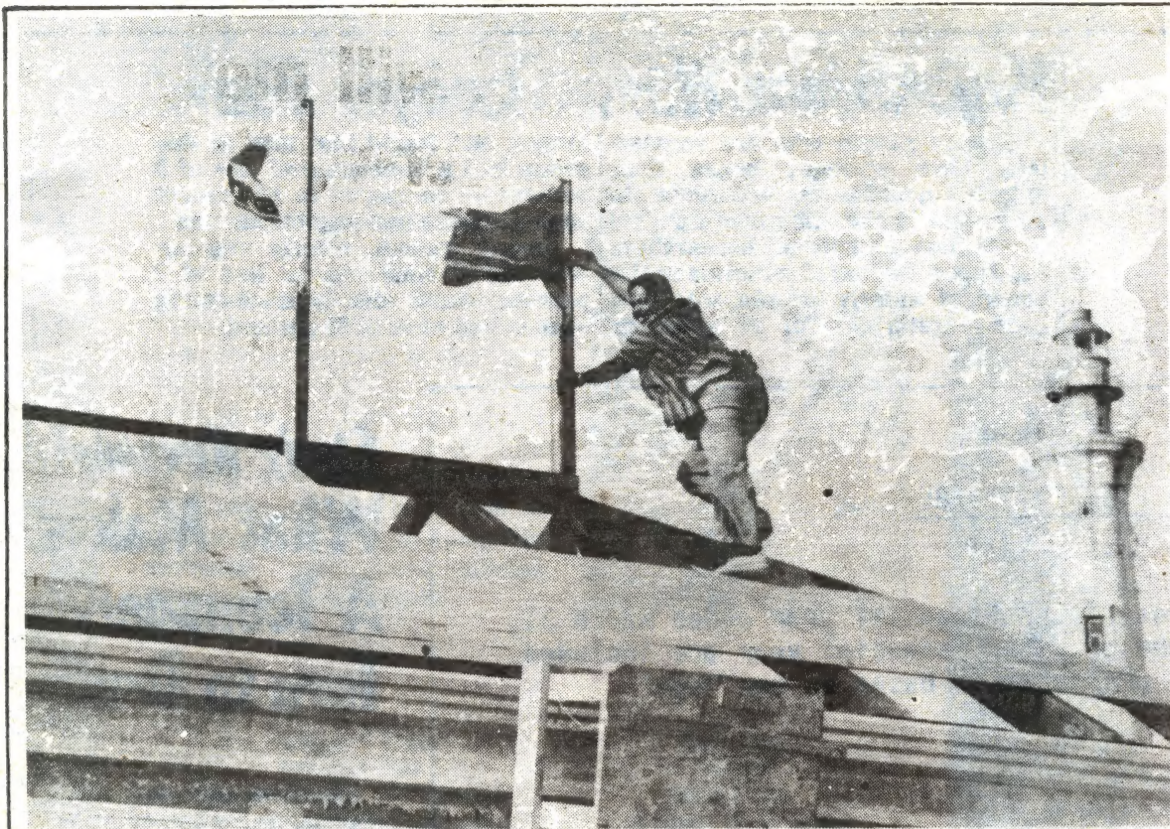
ORANJESTAD—Construction of the "Casa Blanca" Restaurant reached its highest point Saturday and the flags were raised and the beer flowed. The restaurant is being built at Hudishibana, close to the California light house. The project is being financed with aid from the Dutch Government. Mr. Edwin Illidge (hoisting the flag) will be manager of the restaurant which he hopes to open officially on January 6, 1986.
